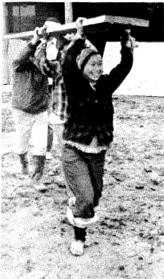
In spite of the rain, we worked on the Village, moving materials, putting up sheetrock and moving tiles onto the roof.
